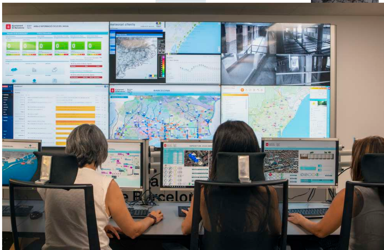
Figure 4: BCASA control centre
