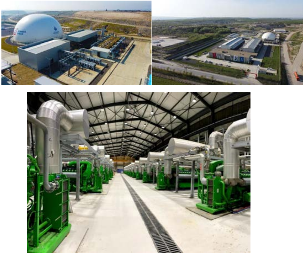
Istanbul Energy Inc. Silivri Seymen Biomass Power Plant
