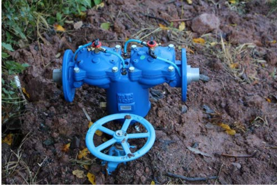
Hydrants Used in Closed Circuit Irrigation Systems
