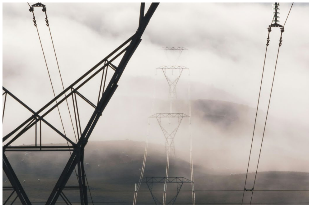
Transmission lines extend into the distance
