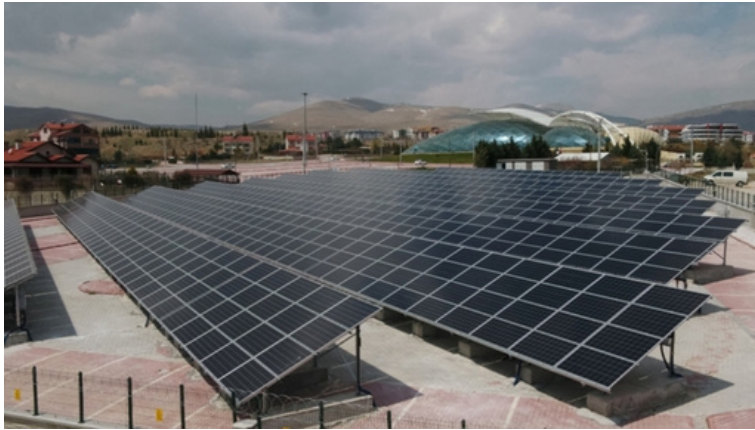
Solar Panel Project (2024)
