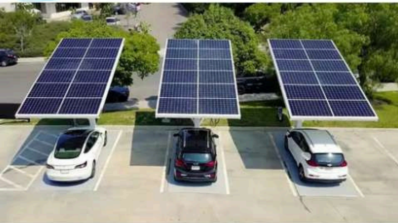
Solar City Project (2024)
