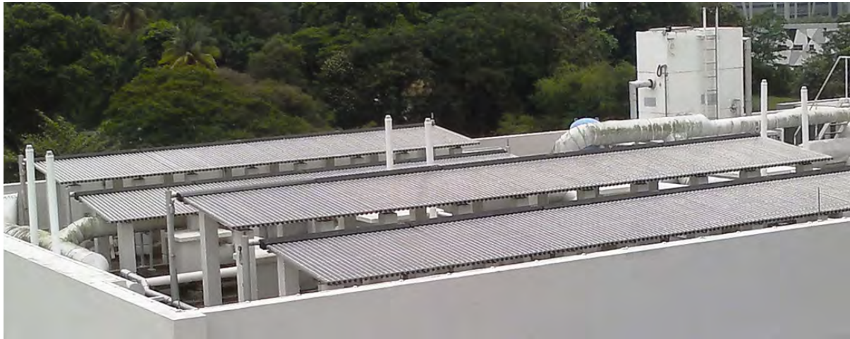
Figure 4.12.5: Solar thermal system installed on building's rooftop
