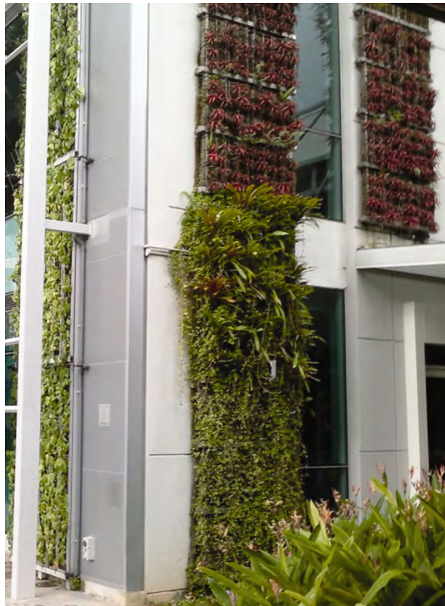
Figure 4.11.10: A green wall helps to reduce the diurnal temperature fluctuation of the building façade.
