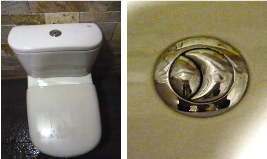
Figure 4.9.4: Toilet with dual flushing cistern.
