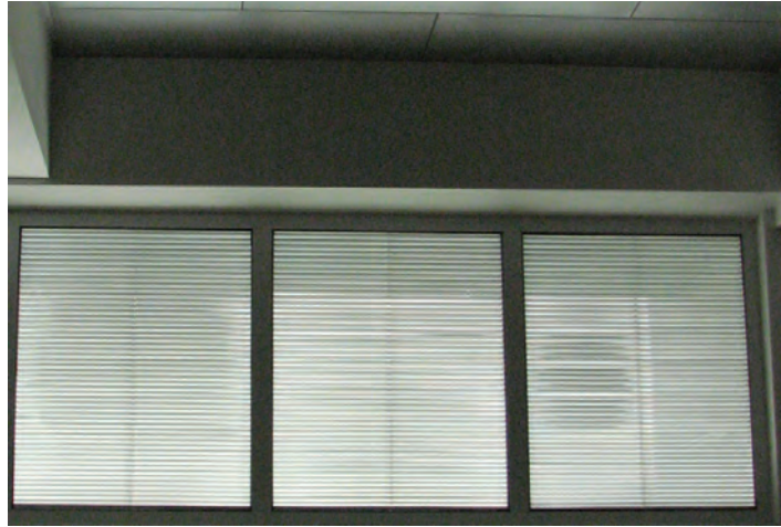
Figure 4.6.3: Diffusive reflective blinds installed within a double glazing façade system
