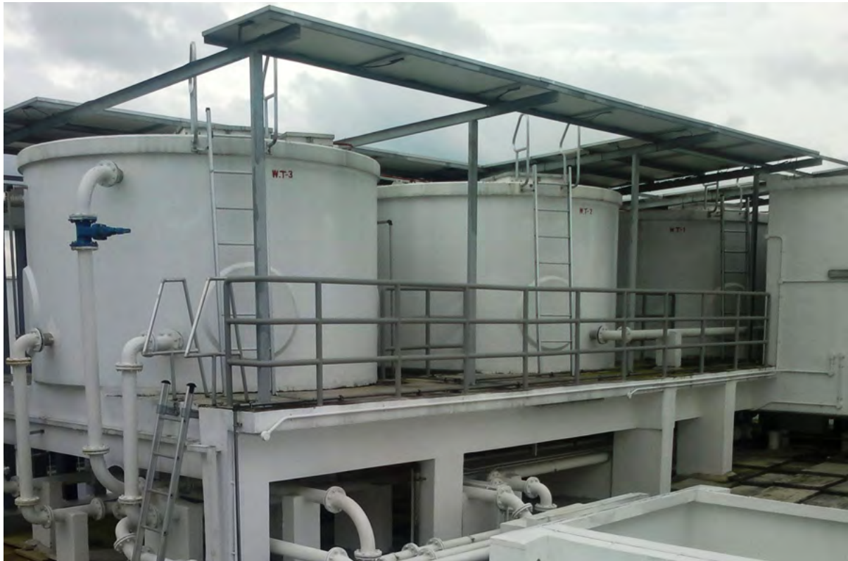
Figure 4.9.7: Rooftop space should be large enough for the water tank and maintenance access
